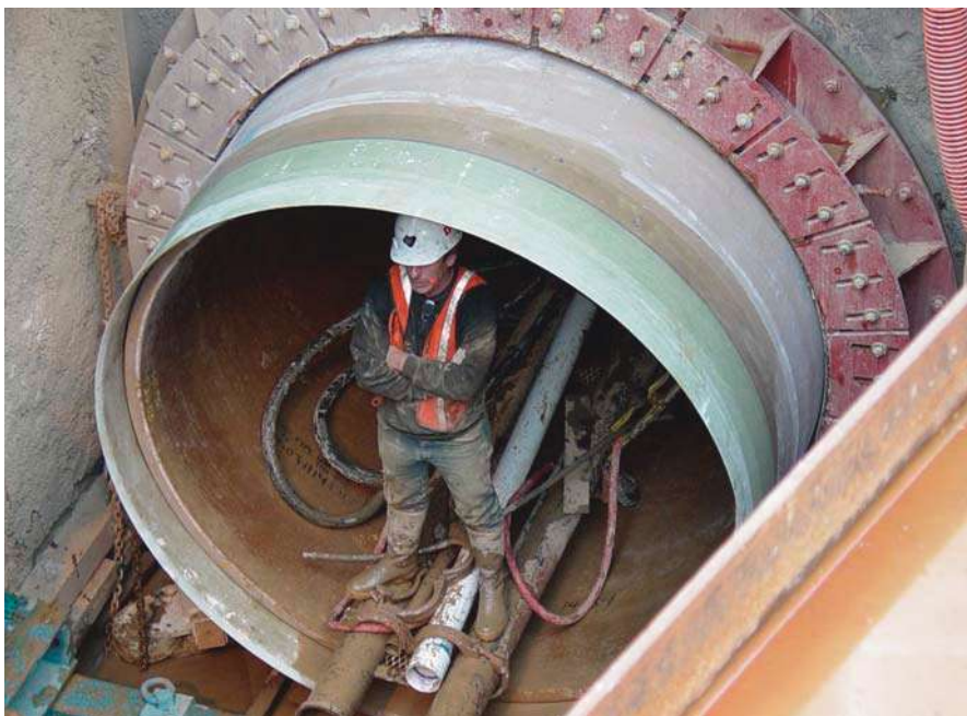
Segmental pipes being continually jacked forward as excavated material is removed via a slurry system.
