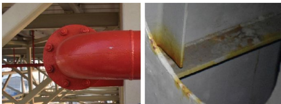
FIGURE 5 Appearance of the \log Z > 7 coatings (left) and of the doubtful coating within the tank (right), after two years of exposure.
