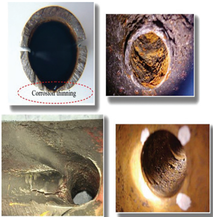
Figure 2 Some failure parts caused by ammonium bisulfide (NH 4 HS).
