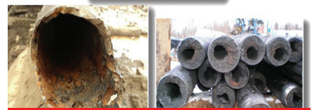
Figure 5 Examples of corrosion caused by hydrogen sulfide.
