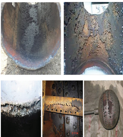
Figure 3 Some failure parts caused by naphthenic acid corrosion.
