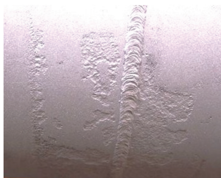
FIGURE 4 External corrosion under solid film-backed, CP-shielding girth weld coating, but no corrosion under the mainline FBE coating.
