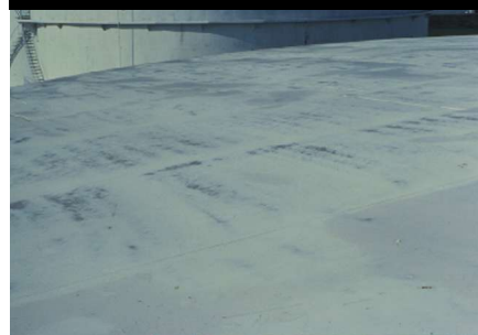
Tank roof showing chalking failure of an alkyd system in a mild environment.
